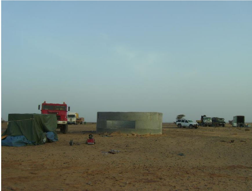
Figure 3. Preparations have been made to test out a new well recently drilled near Afraijat Albashir, Western Sahara, May 3, 2008. Photo by Alice Wilson
