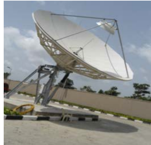
FIG. 12 7.6M CO-LOCATED ANTENNA SYSTEM
